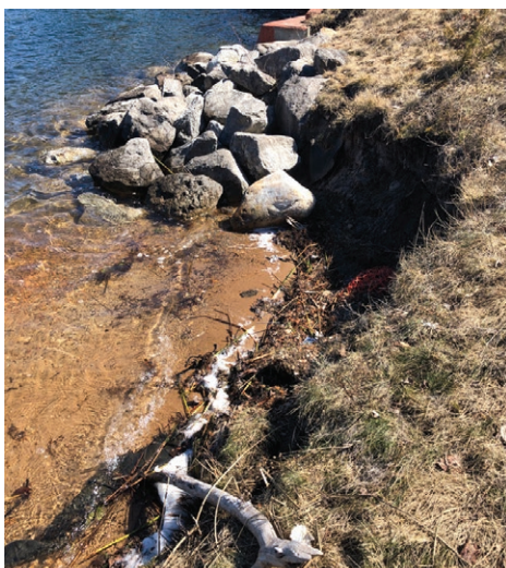
An installation where uniform rock size and lack of attention to the end of the revetment actually accelerated erosion.
